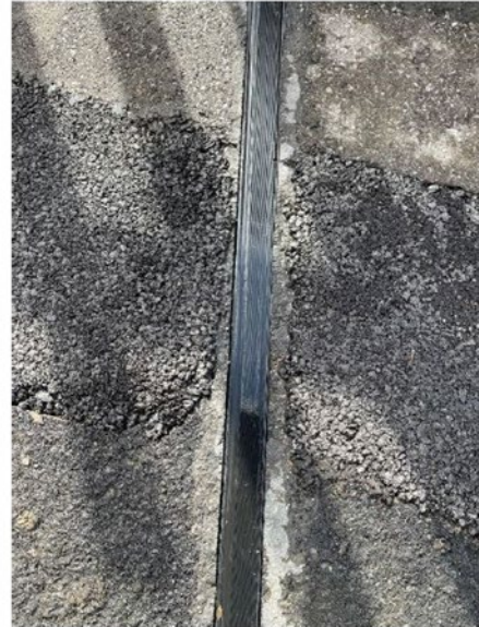
Reinstating the pavement up to the edge of the Kerbo Charge channel
